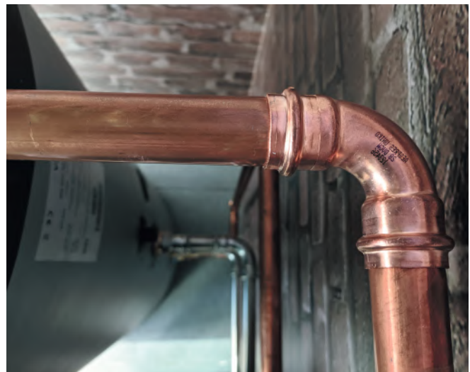
Figure 16 - aesPRES UNIKO - Heating installation
